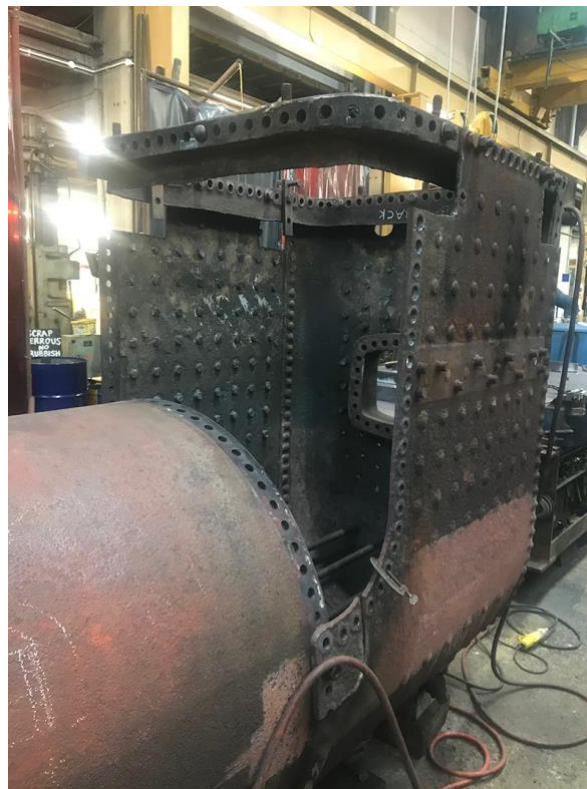
The boiler with the throatplate and inner firebox removed
